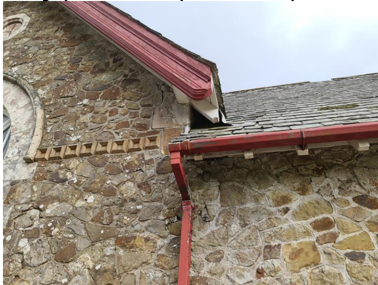
Photograph 3: Example of the exploitable areas where roof pitches key into each other
